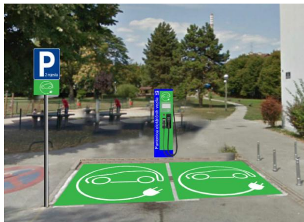
Charging station Trešnjevka
