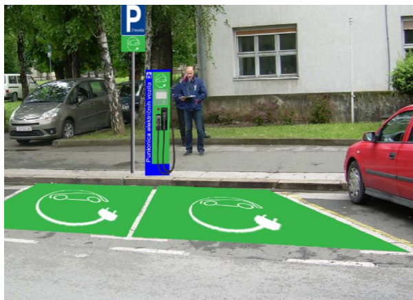
Charging station Črnomerec
